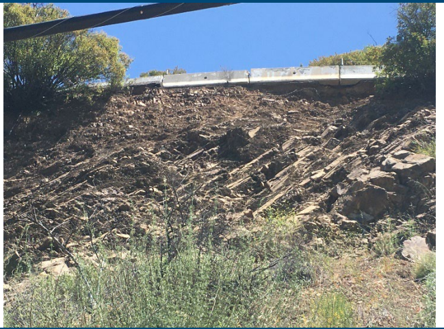
Undermined Matilija Canyon Road ~MP 0.42
