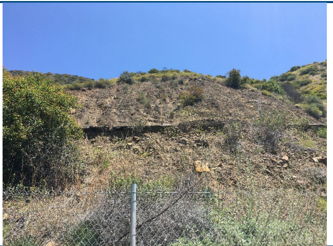
Undermined Matilija Canyon Road ~MP 0.63, looking up from lower access road
