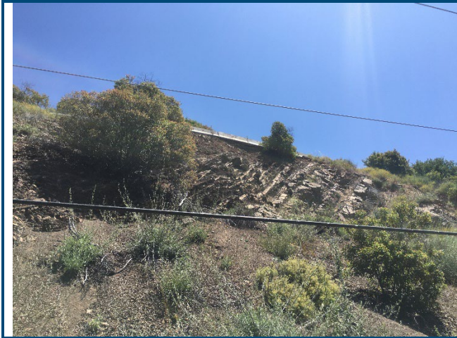
Undermined Matilija Canyon Road ~MP 0.42
