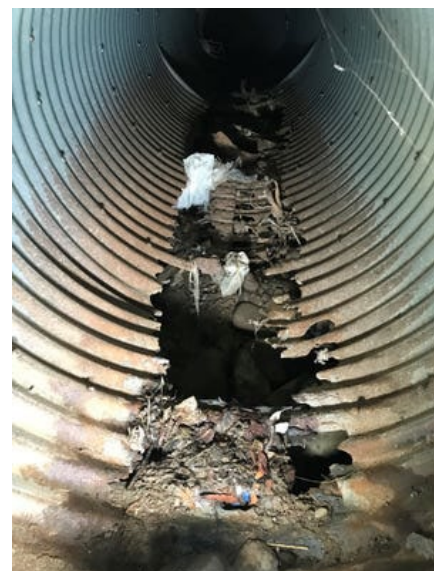
A broken pipe led to several sinkholes opening up in a Ventura neighborhood. CONTRIBUTED PHOTO/VENTURA COUNTY PUBLIC WORKS
